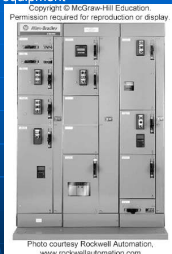
Figure 3-16 Typical motor control centers
